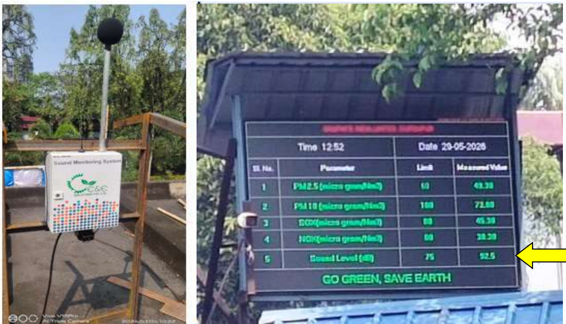
For EC compliance Ambient Noise level Monitoring Station Installed – & Commissioned
